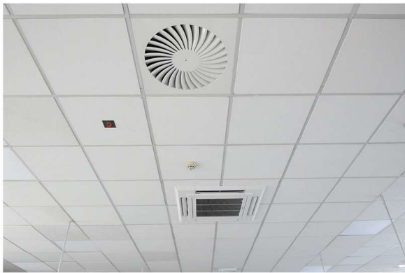
New ceiling and ventilation Units. Ward 5. (Unused newly created Covid Ward) Lancaster Royal Infirmary. 17th June 2020
